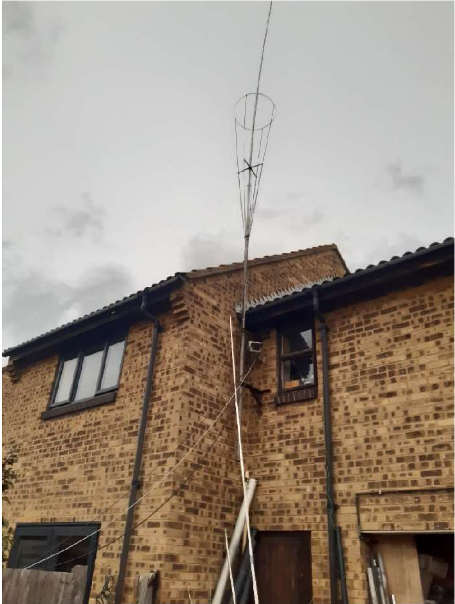
The wall mounted antenna on the rear elevation.
